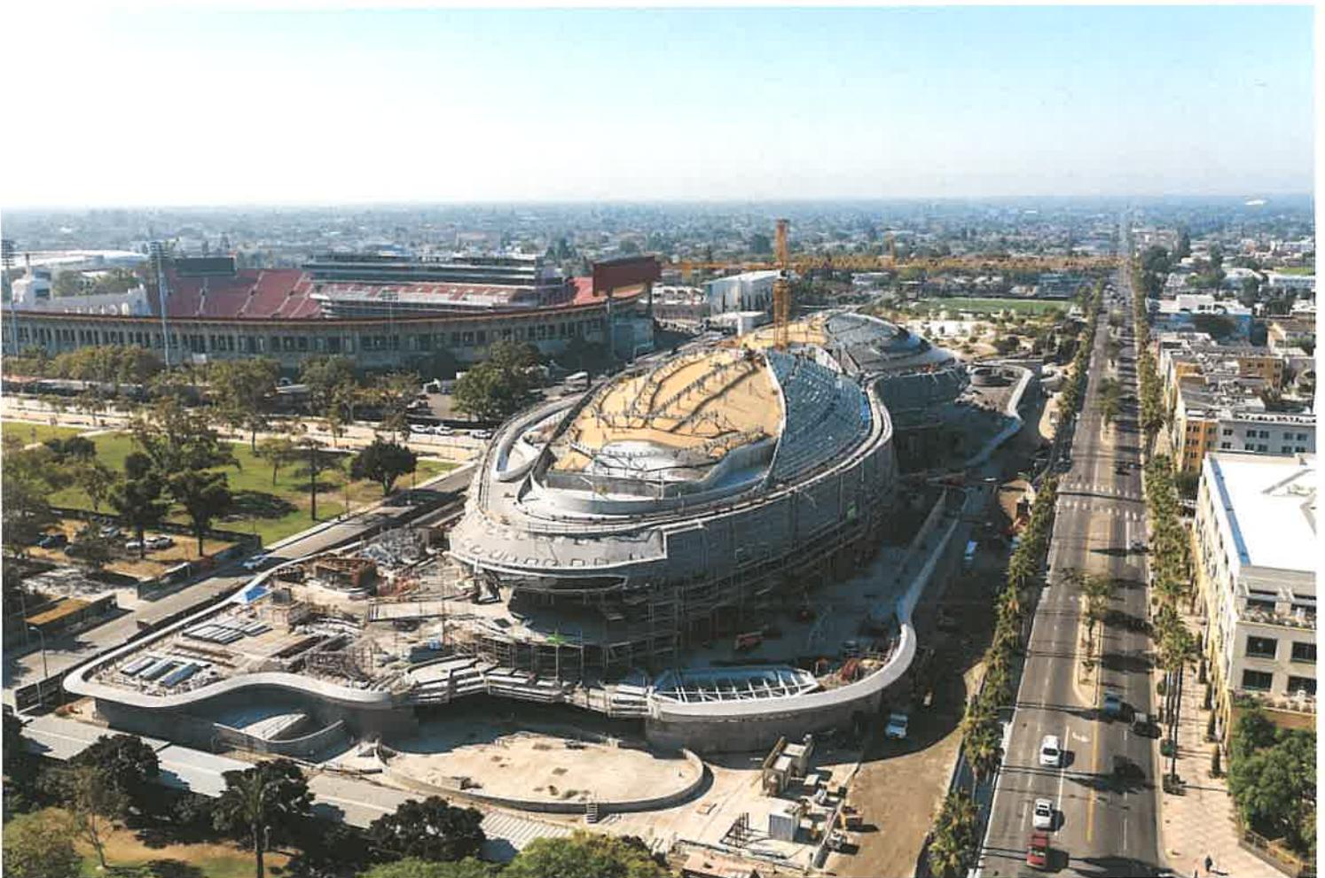
The under-construction Lucas Museum of Narrative Art, in June, looking south from Vermont Avenue. (Photo by Hunter Kerhart; ©2022 Lucas Museum of Narrative Art.)
