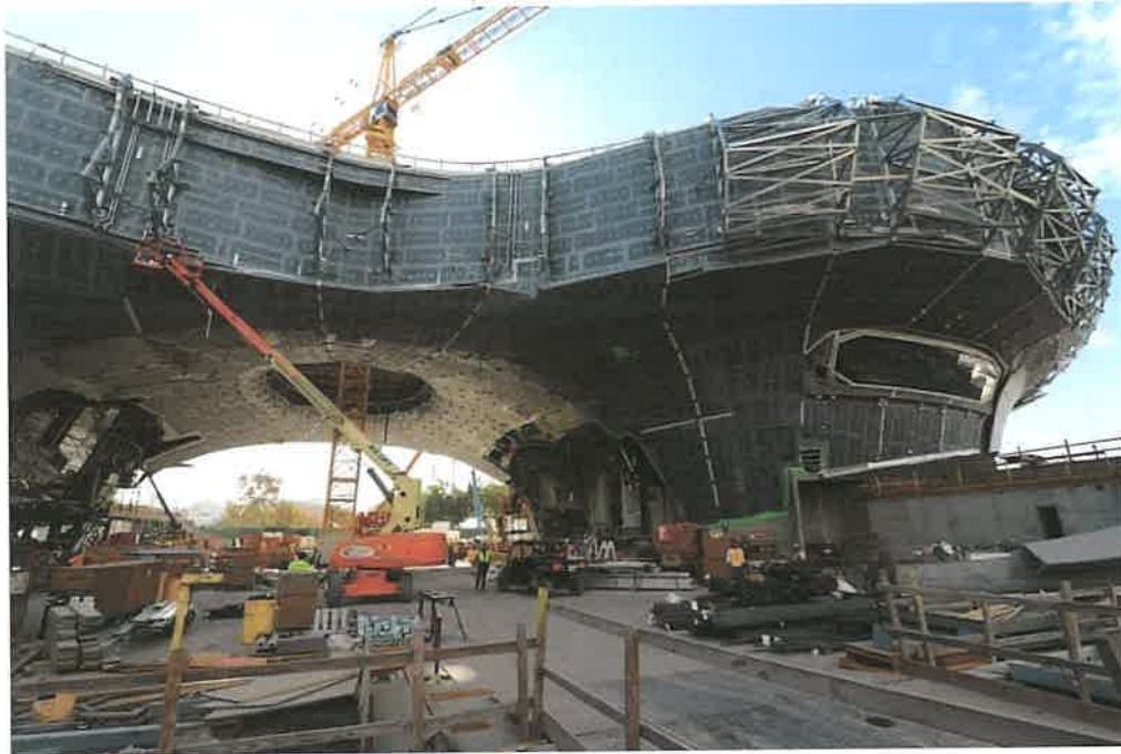
Lucas Museum plaza construction, August, 2022. (Photo: Roberto Gomez, USC School of Cinematic Arts. All rights reserved. ©2022 JAKS Productions. )
