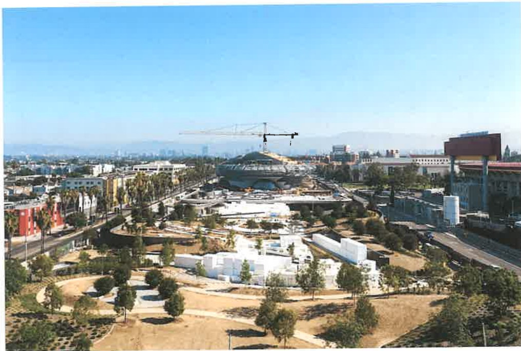
Lucas Museum park and building construction, looking north, June 2022. (Photo by Hunter Kerhart; © 2022 Lucas Museum of Narrative Art.)
